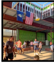
September 2, 2019 Signing the Beams All of the St. Catherine parishioners and all the workers who contributed to building St. Catherine of Siena were invited to sign their names on the final beams.
